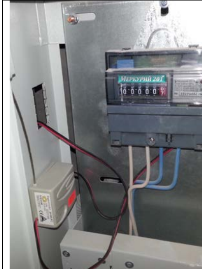
Electricity - 2 metering device
