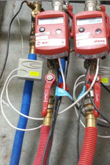
Heat metering - two meters on radiomodule
